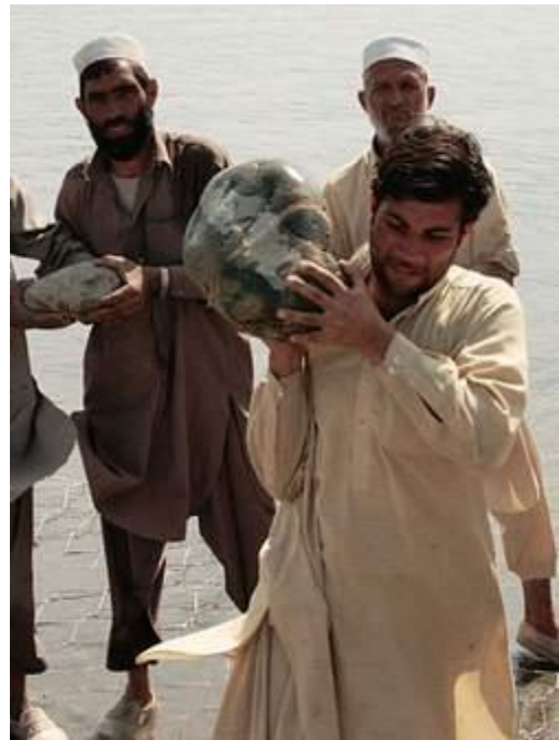
Every stone added to the wall is one step further to some more secure agricultural land.
